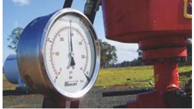
WELL HEAD PRESSURE GAUGE
